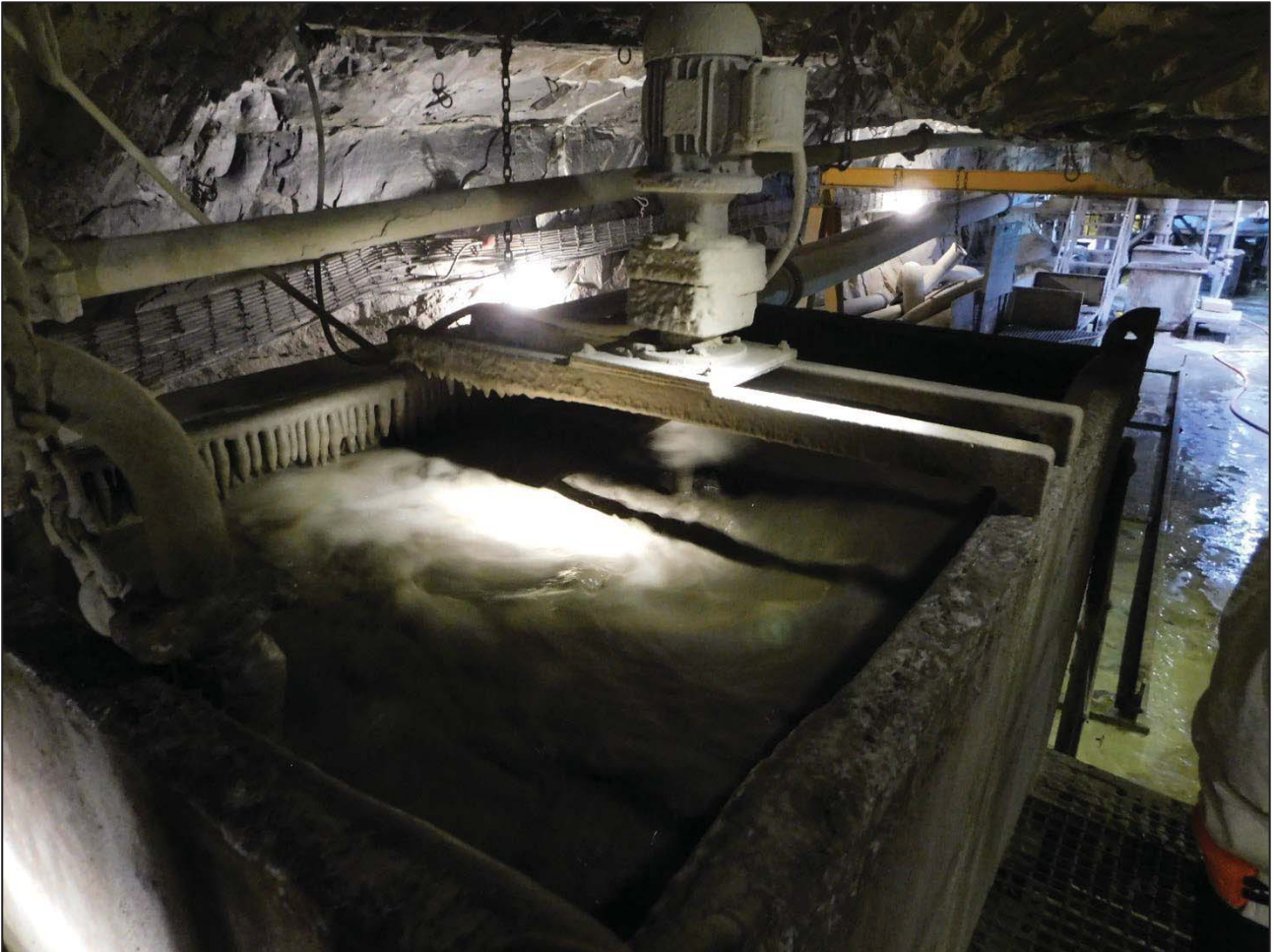
Figure 3-11 Example of an underground mine dewatering scheme where water is channelled to a central location and removed from the mine with large pumping systems.
