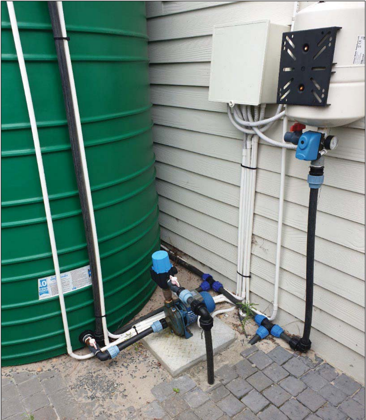
Figure 3-2 A private groundwater scheme at a household where a borehole is used for non-potable, domestic supply. The borehole headworks can be seen with a large JoJo tank for storage, as well as a small filter and treatment system installed on the wall.
